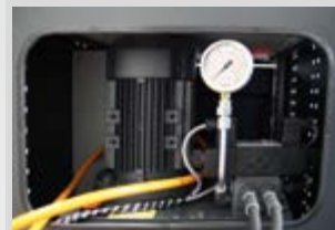
Dual-circuit hydraulic unit in cabinet base
