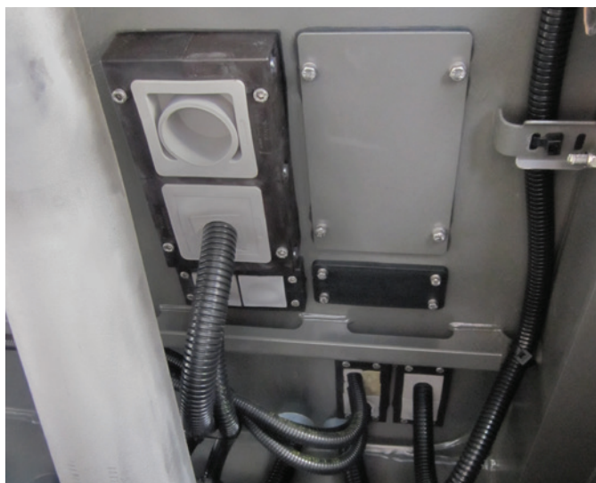
KEL-JUMBO 2 / KEL 24|x Routing of conduits and large cables between vehicle body and chassis
